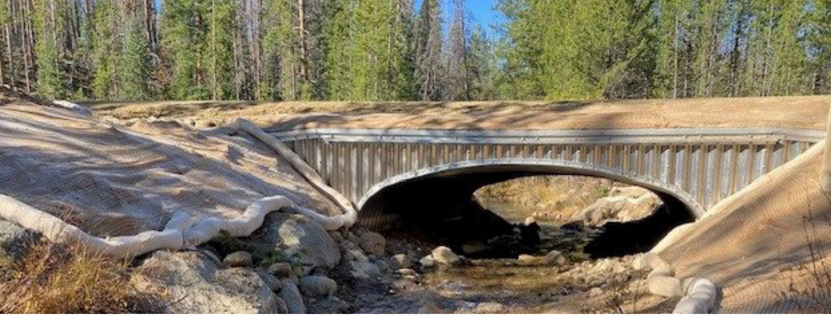
Cabin Creek culvert replacement was completed in October 2021. After construction, the area was restored with native grasses. Special netting was installed to hold the ground in place until grasses re-establish around the site. Photo courtesy of Denver Water
